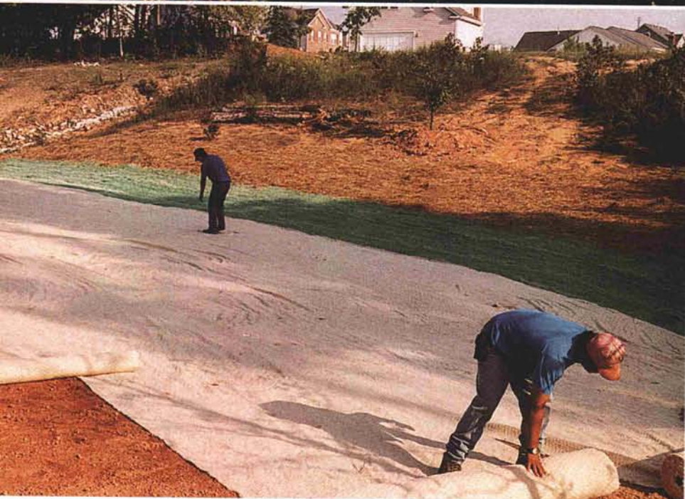
Workers install flexible revegetation blankets, which are designed to prevent under-blanket washouts and seed migration.
