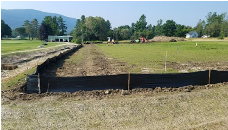
Figure 1-3. The drainage ditch was over-seeded with a erosion control mat, hay bales were placed inside the drainage ditch, and the entire project was surrounded by a silt fence prior to any construction taking place within the project.
