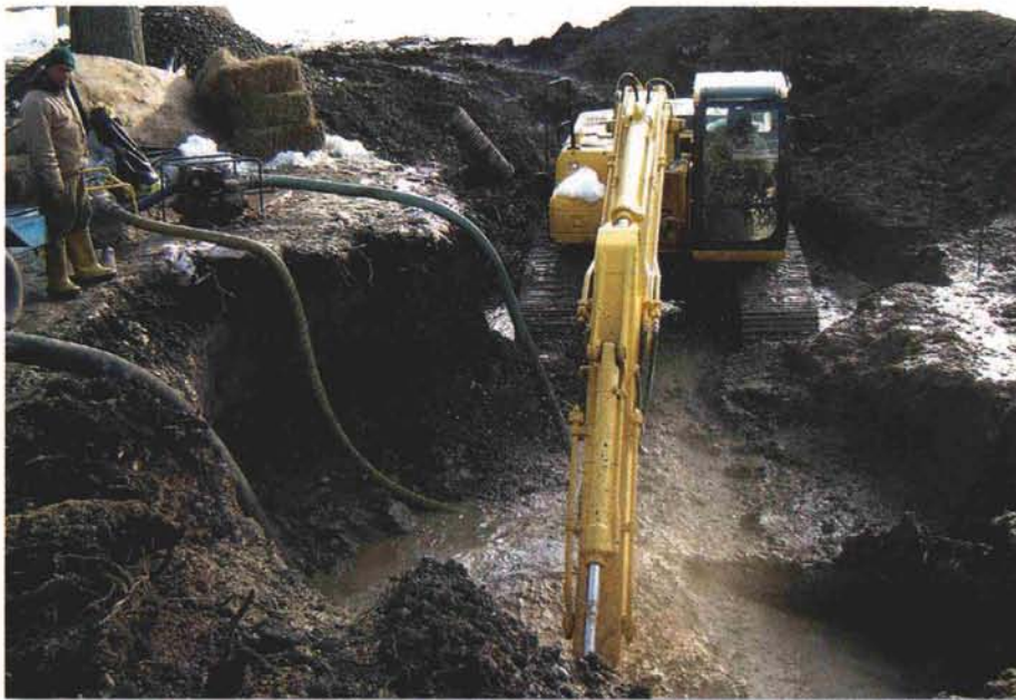
The team at the The Millbrook Club excavates for a pump chamber to be installed.
