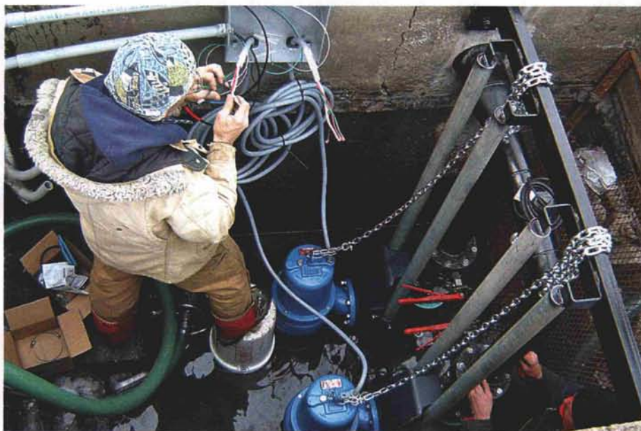
In the middle of a mild and wet winter, the crew installs pumps inside the new chamber.
